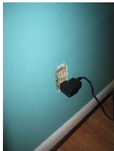
#36 Missing cover plate.
