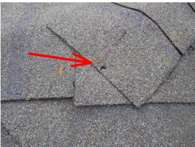
#23 Exposed roofing nail and hole should be sealed.
