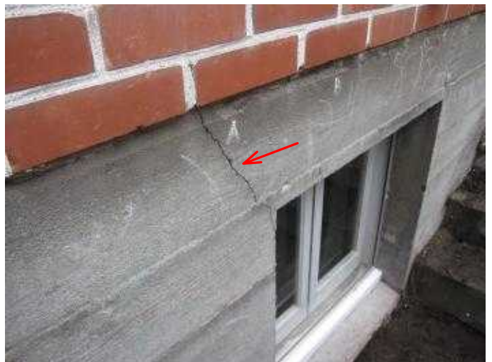
#6 Minor settling crack in foundation on North side. Should be sealed.
