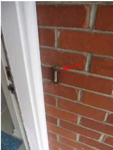
#9 Rear doorbell non-functioning.
