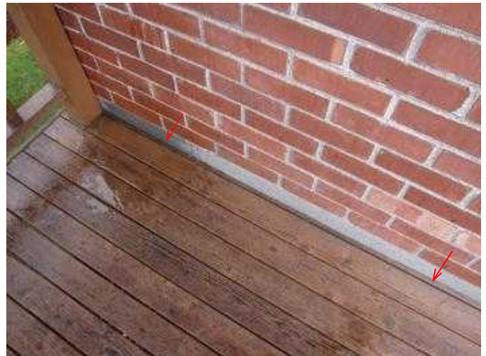
#10 Flashing should be installed at deck to house junction.
