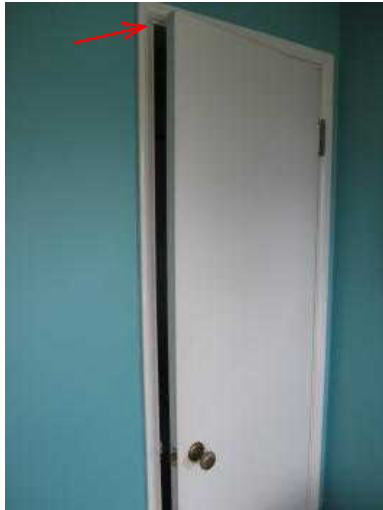
#37 Closet door sticks in jamb.
