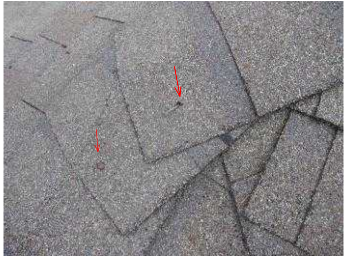
#20 Exposed roofing nail and protruding nail should be sealed.
