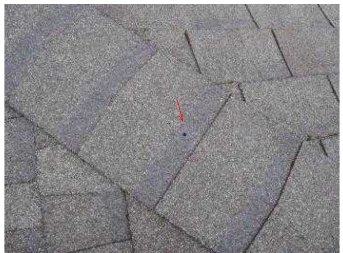
#18 Nail hole in roof should be sealed.
