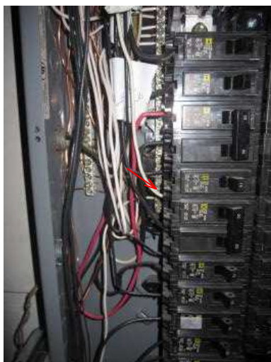
#41 Neutral wire used as hot wire.
