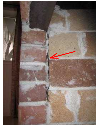
#40 Missing mortar in basement fireplace.
