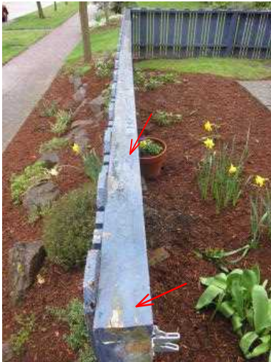
#3 Fence system has minor rot and peeling paint.
