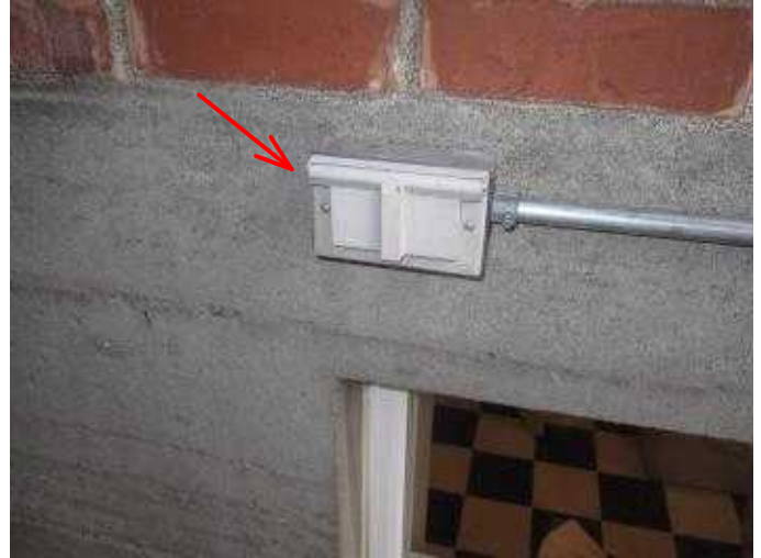
#14 GFCI outlet on South exterior no tripping when tested.
