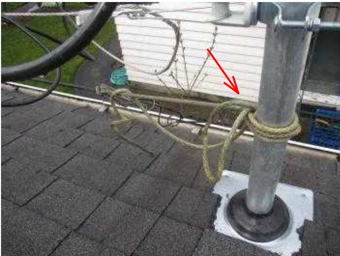
#21 Telephone lines should be permanently secured to mast.
