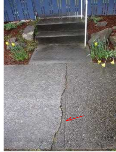
#2 Minor settling and crack in front walkway
