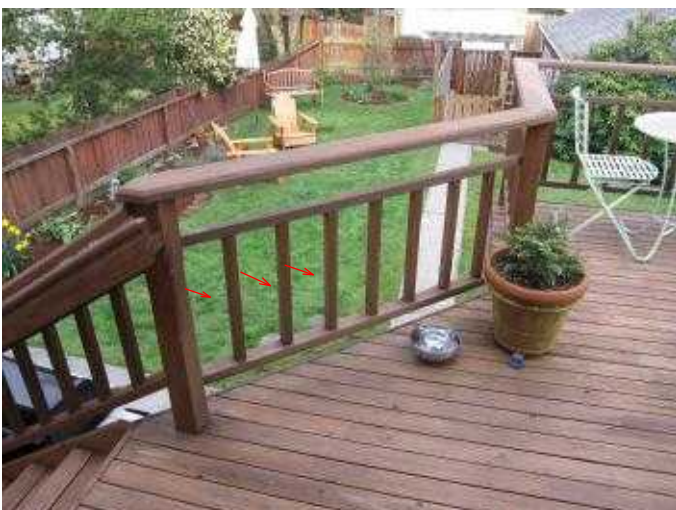
#11 Balluster spacing too wide. (safety)
