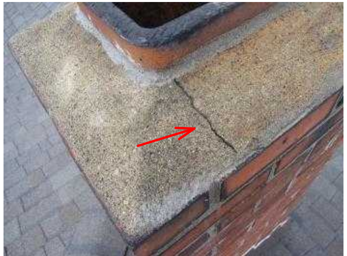
#22 Crack in North chimney crown should be sealed.
