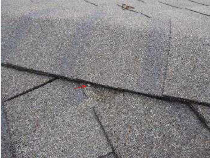
#25 Nail heads should be sealed.
