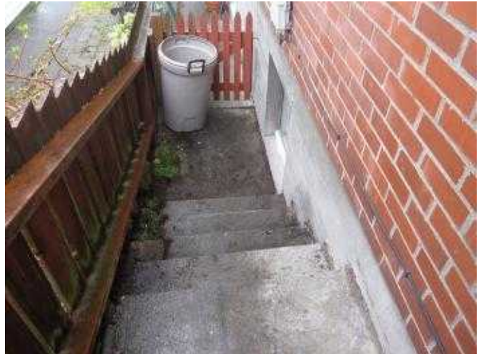
#4 No handrail on North steps.
