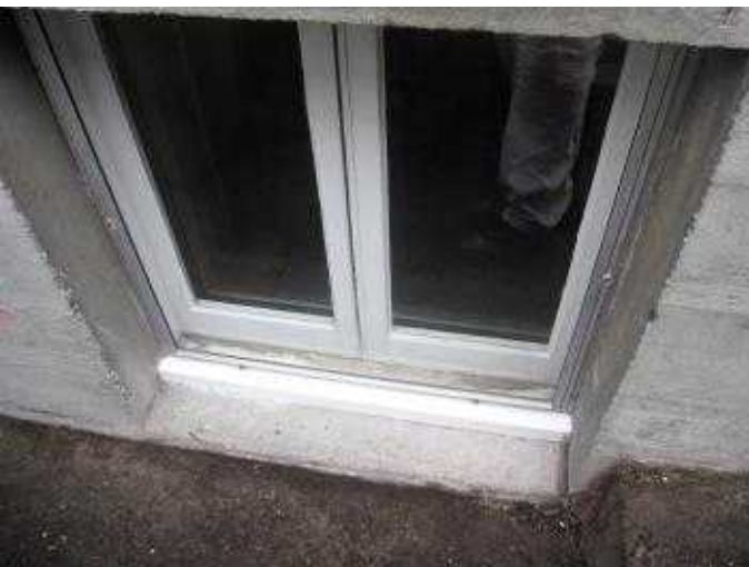
#5 Storm window on North basement window should be tempered. (safety)
