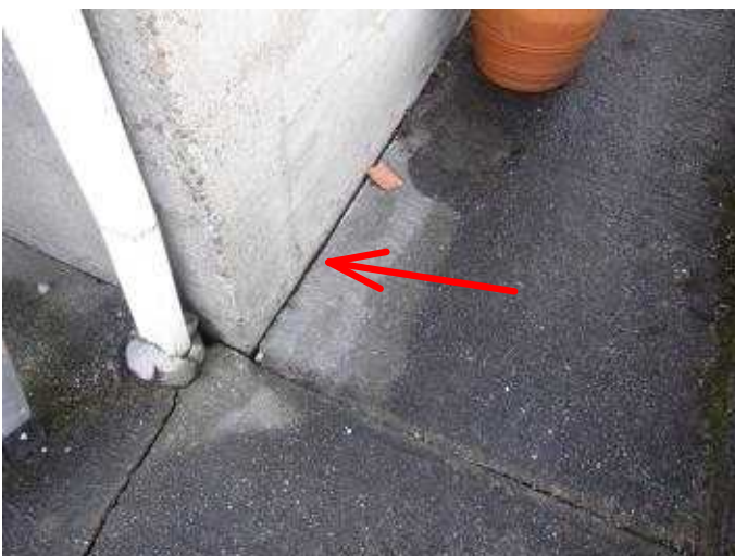
#29 Crack should be sealed where walkway meets foundation.
