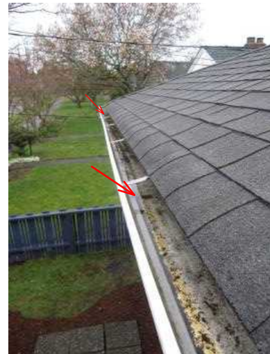
#16 Minor pooling of water in gutter system.
