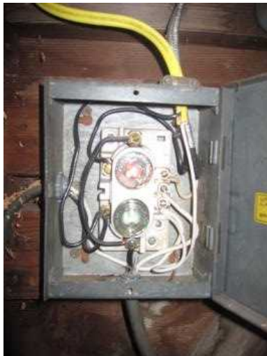
#27 Knob and tube junction box should be upgraded in garage.
