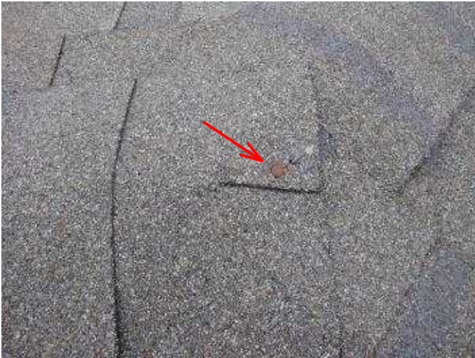
#19 Exposed roofing nail should be sealed.
