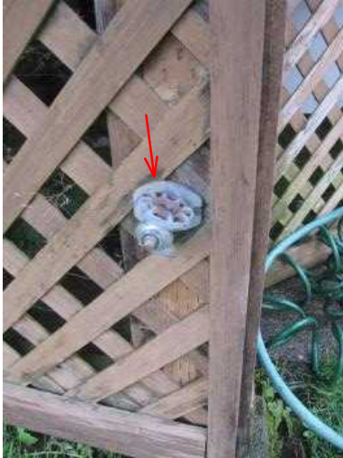
#13 Abandoned hose bib no longer functional.
