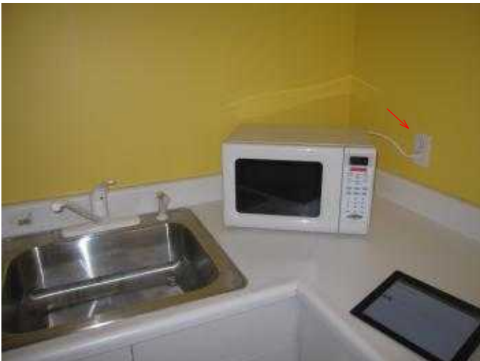
#39 Outlet in utility room should be GFCI protected.
