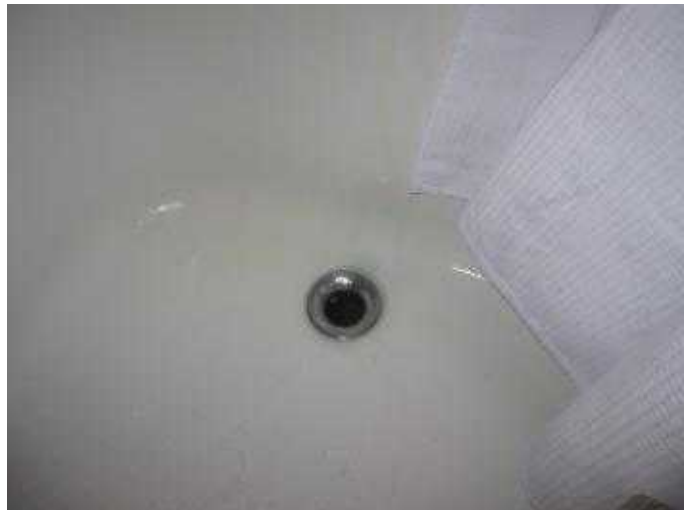
#34 Upstairs bathtub missing stopper.
