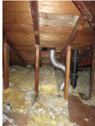
#32 Bathroom vent duct should be secured to outside.
