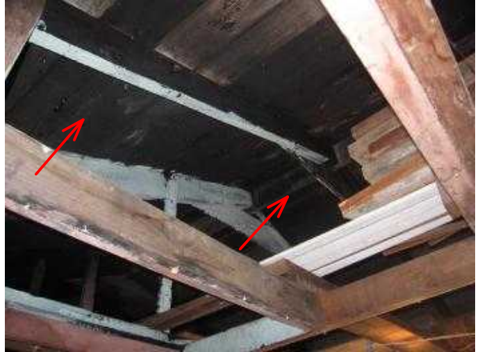
#26 Signs of previous fire in detached garage.
