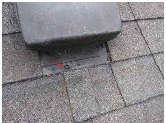
#24 Nail heads should be sealed.
