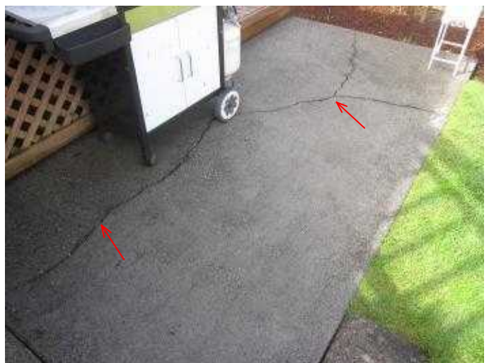
#30 Moderate cracking in patio slab.
