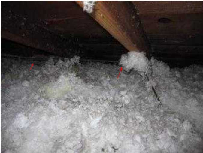
#31 Original knob and tube present in attic and buried in insulation.
