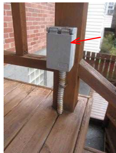
#12 GFCI outlet on deck not tripping when tested.
