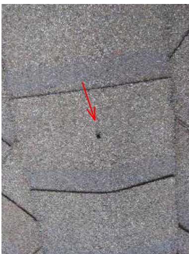
#17 Nail hole in roof should be sealed.
