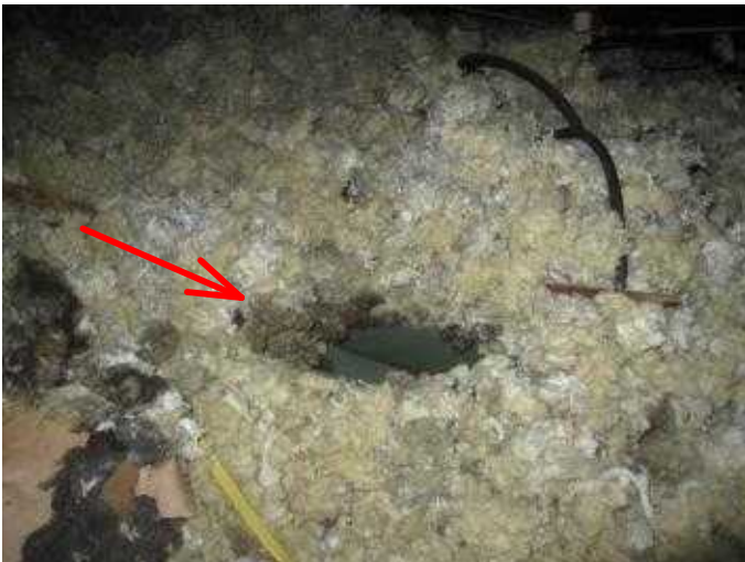
#33 Kitchen exhaust fan vents directly into attic.
