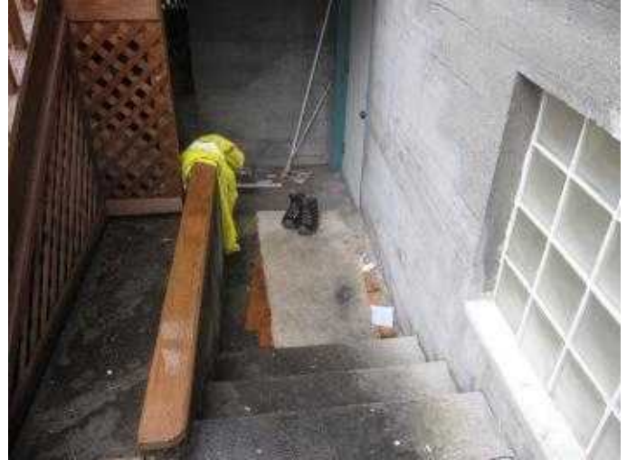
#8 No handrail on steps leading to basement.
