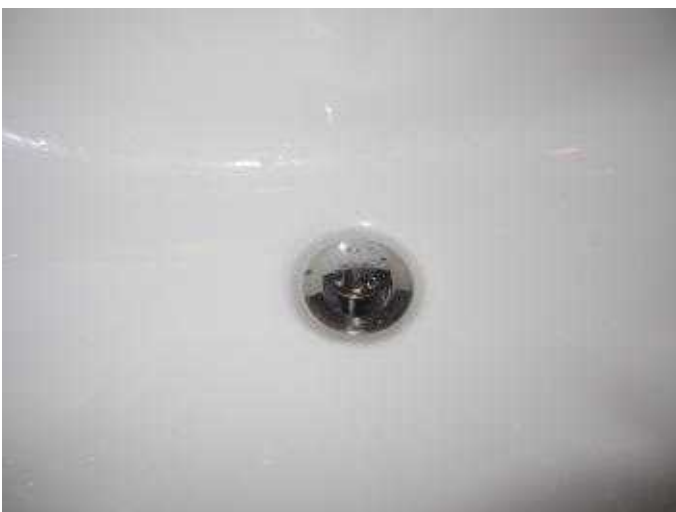
#35 Upstairs sink stopper non-functioning.
