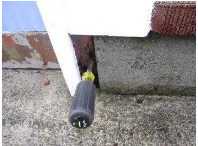
#28 Moderate rot in garage side door jamb.
