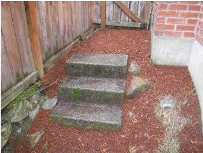
#15 No handrail on South steps.
