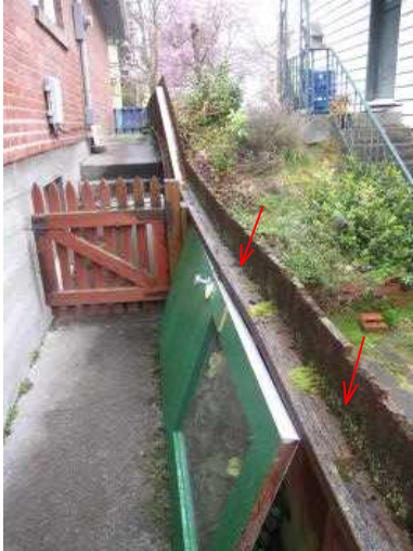
#7 Fence system shows signs of rot.
